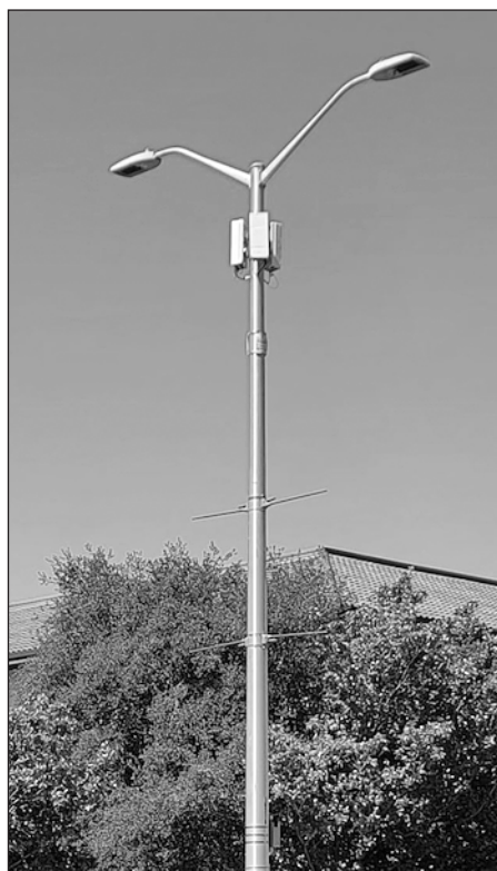
If you travel anywhere in Fremont, you might have noticed small boxes attached to the top of light poles around the city. These boxes are small wireless facilities,
