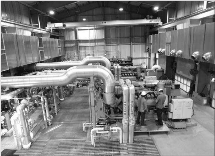
Lee and Fulkerson check cogeneration engines, which transform methane gas into energy to run USD's treatment plant
