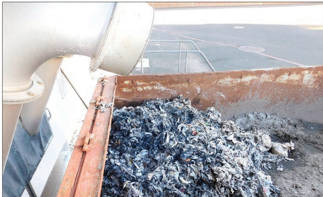
Wipes removed from wastewater at USD's treatment plant
