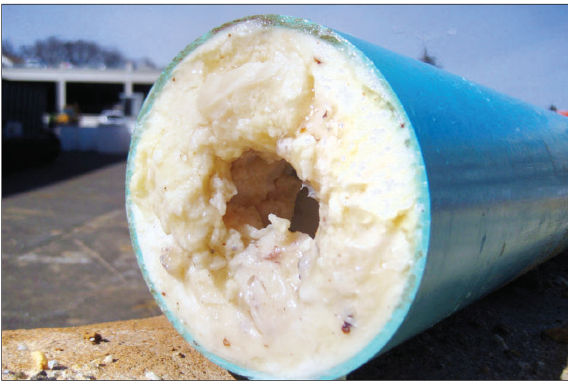
Grease buildup in a sewer line
