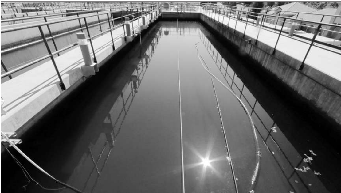
Water is allowed to slowly pass through settling tanks like this where naturally occurring sediments are extracted.
