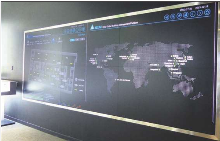
Delta Building Management software on Delta display screens
