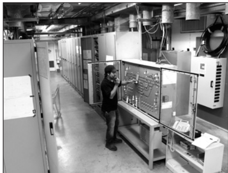
Train Control Electronic Technicians are in constant contact with the BART Operations Control Center.
