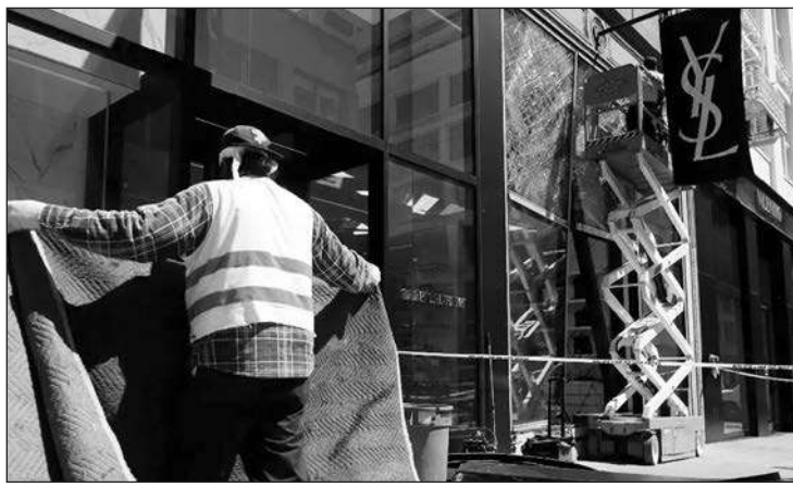
A work crew removes broken windows at a Yves Saint Laurent store in San Francisco after a robber backed a car into a window of the store in San Francisco's Union Square then jumped out of the car and burglarized the store, according to police. Credit: AP Photo/Jeff Chiu
