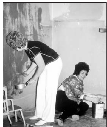
Catherine Mozzetti (at right), works hard on the Shinn House restoration (1970s).
