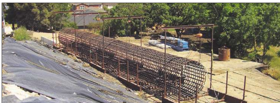
New bridge construction is progressing south of the existing bridge. This CIDH rebar cage will be inserted into drilled hole and filled with concrete.
